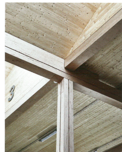
CLOCKWISE FROM FAR LEFT, A SPECTACULAR SERIES OF 16 ROOF LIGHTS SET AT 40-DEGREE ANGLES FUNNELS IN SOFT, NORTH LIGHT; THE BEECH LAMINATE-VENEER LUMBER ENABLES BEAMS AND COLUMNS TO HAVE SMALLER CROSS-SECTIONS THAN SOFTWOOD GLULAM, PROVIDING THE STRUCTURE WITH A LIGHTER AND MORE ELEGANT APPEARANCE; ARCHITECT AND CHIEF ADVISOR MARTIN FRANCIS
