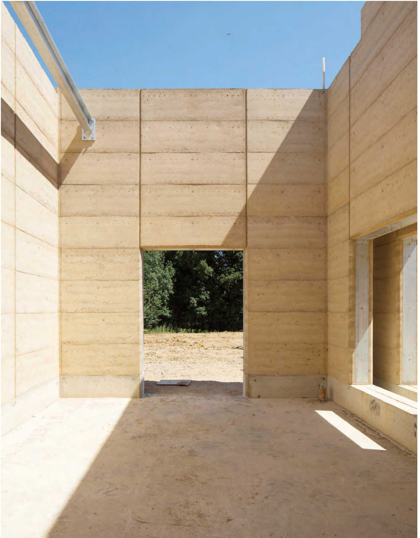
Above Prayer hall interior with rammed earth walls, which will remain exposed
